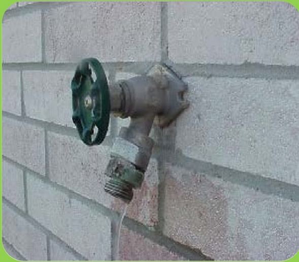
Exterior Water Faucet
