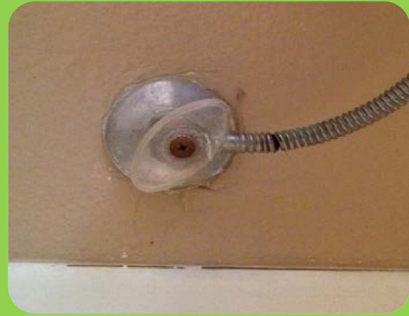
Line Appears Damaged
