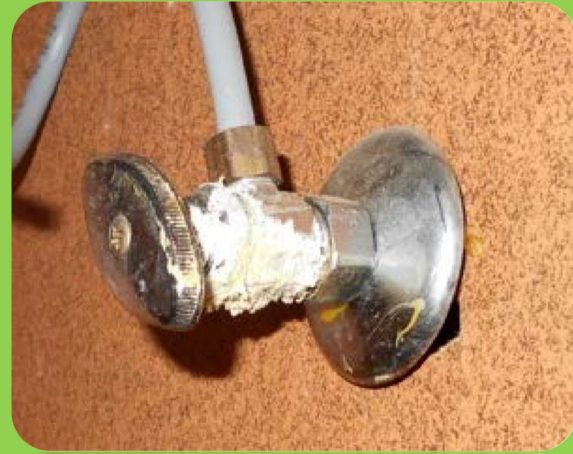
Valve Appears Damaged
