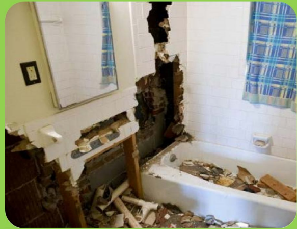
Vandalism: Walls Opened for Copper
