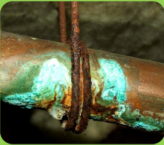
Corrosion: Damage to Copper Line
