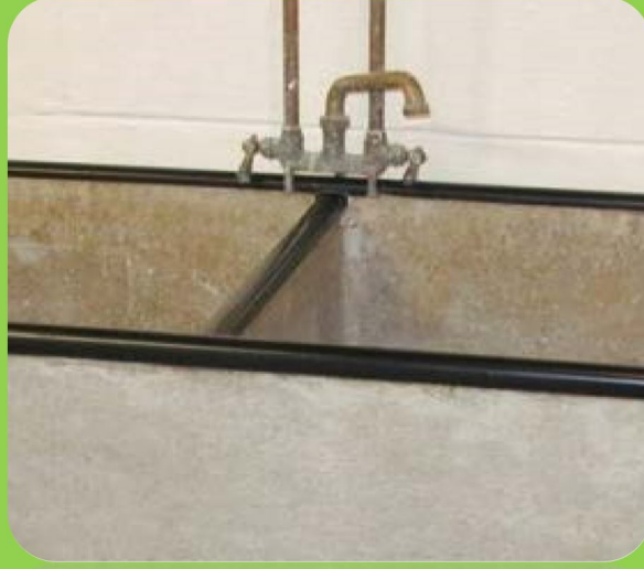
Interior Water Faucet
