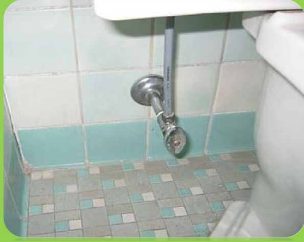
Toilet Shut Off Valve
