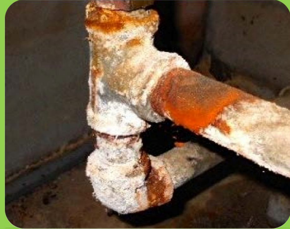
Joints Appear Damaged
