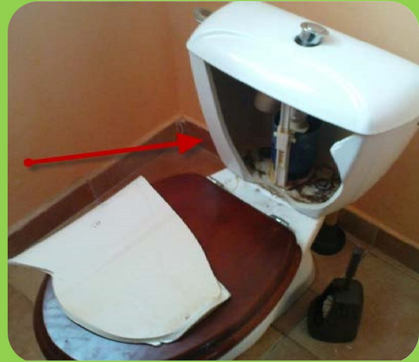
Freeze: Cracked Toilet Tank
