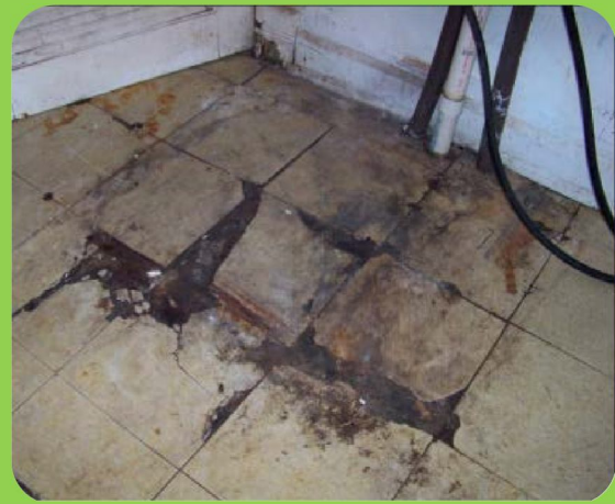
Floor Appears Water Damaged
