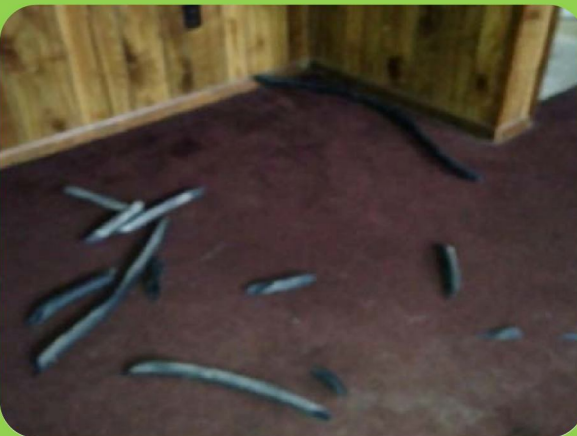
Vandalism: Pipe Insulation on Ground
