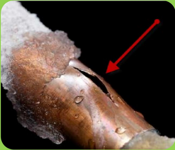
Freeze: Fissure in Copper Line
