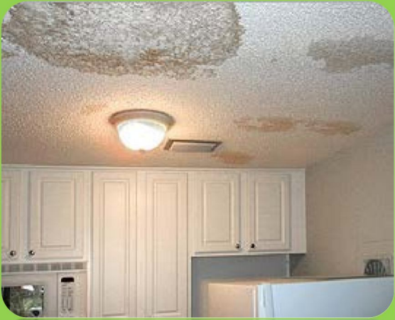
Ceiling is Wet/Stained from Damage
