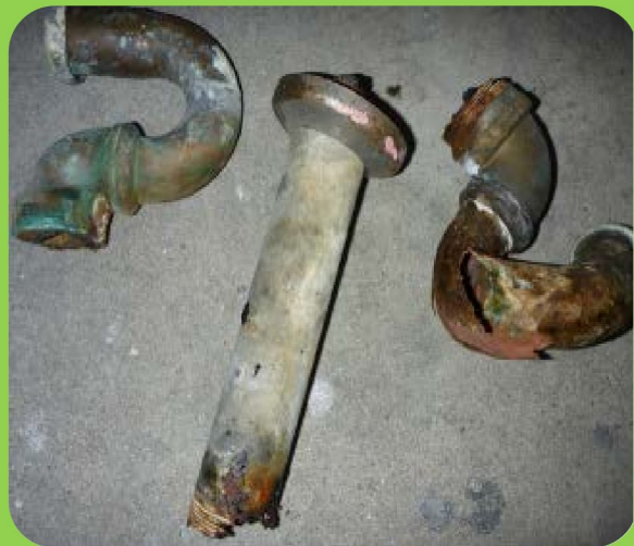
Corrosion: P-Trap Damaged
