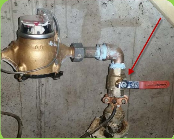
Water Meter Shut Off Valve
