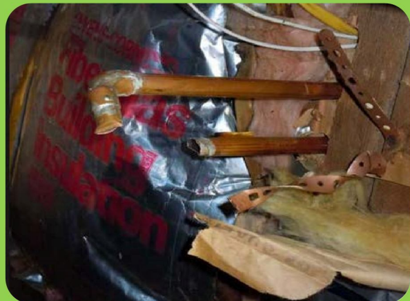
Vandalism: Pinch Cut to Remove Copper
