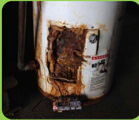
Corrosion: Damage to Heating Element
