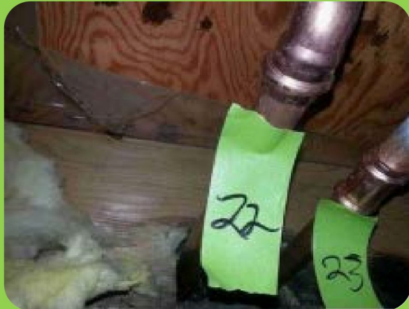
Damaged Copper Properly Marked
