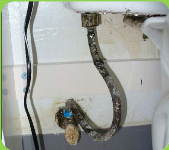
Corrosion: Supply Line Damaged
