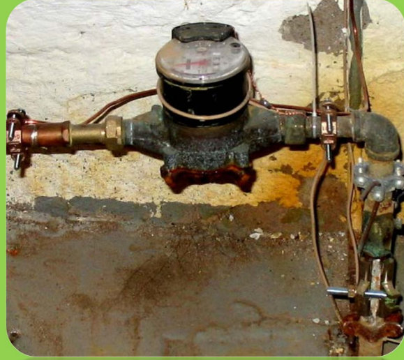
Interior Water Meter
