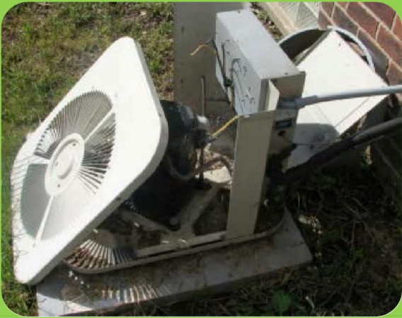
Vandalism: Copper taken from ac unit
