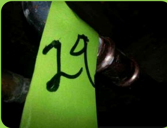
Damaged Copper Properly Marked
