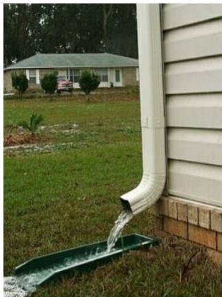
Splash pad is diverting water away from the foundation and protecting the ground from eroding causing a hole or damage to the landscape
