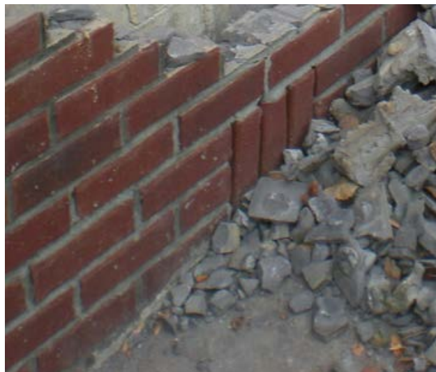
Crumbling Decorative Brick
