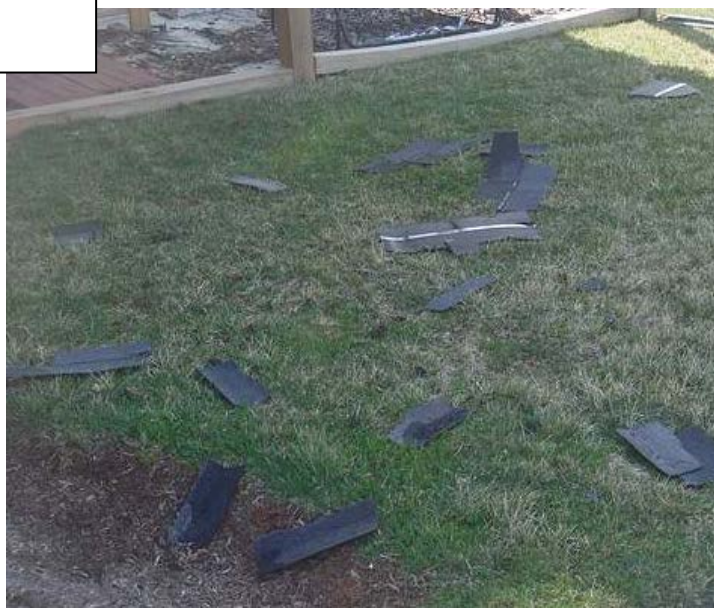
Damaged Shingles on Ground
