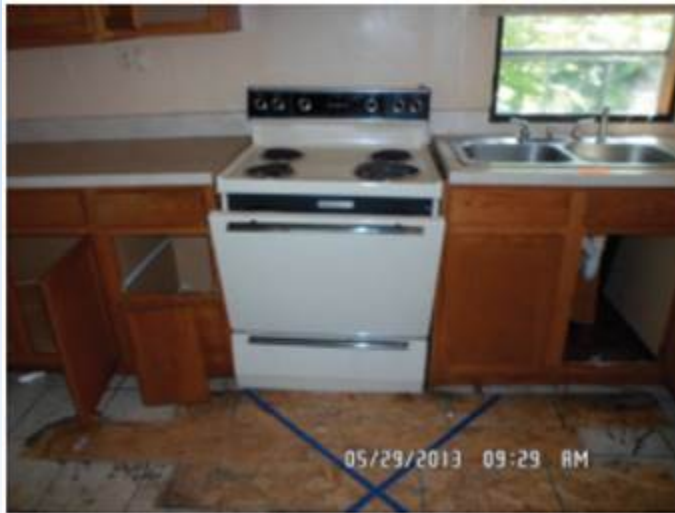
Appliances fallen through rotten floor
