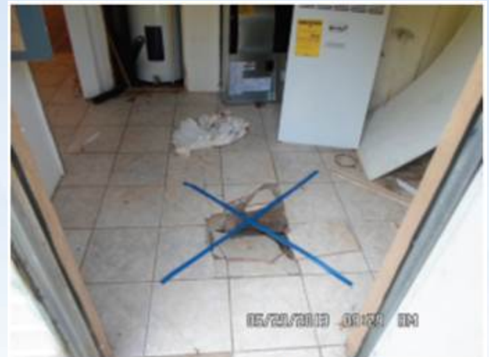
Rotten floor in utility room
