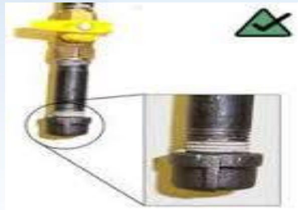
Cap all gas lines.
