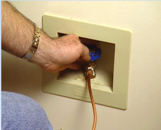
Cap kitchen water lines.
