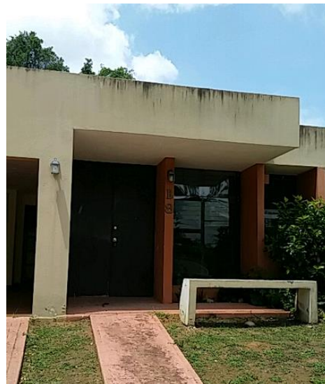
POOR FRONT OF HOUSE PHOTO
