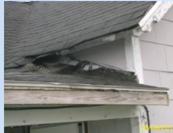
6/8/13 Roof damage photo submitted by HUD
