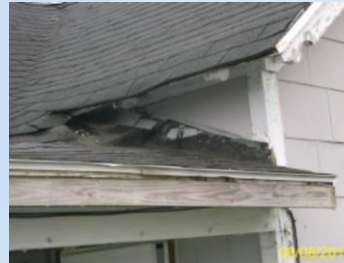
6/8/13 Roof damage photo submitted by HUD
