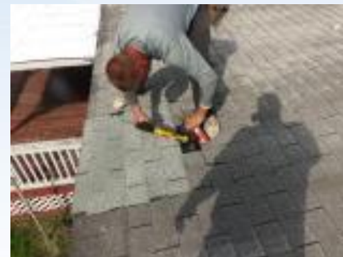
Improper – Patch is on top of old roofing creating a bump. Shingles are not feathered into existing roofing.
