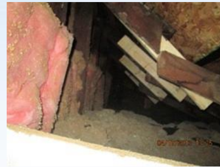
Improper Structural Repair
