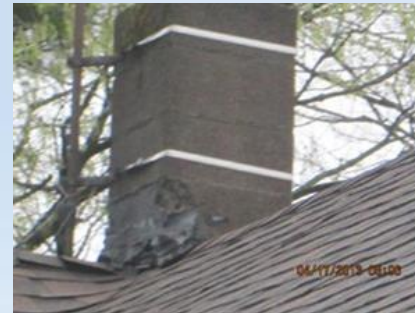
Improper Chimney Flashing
