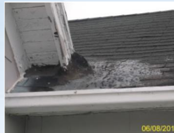
6/8/13 Roof damage photo submitted by HUD
