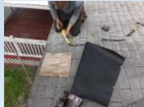
Improper – Felt paper being glued down with roof cement
