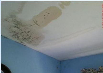
Interior water stains and discoloration on ceiling
