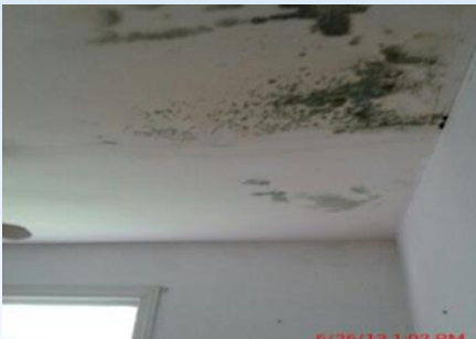
Interior water stains and discoloration on ceiling
