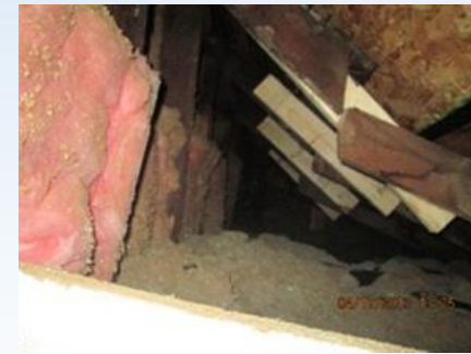
Improper Structural Repair
