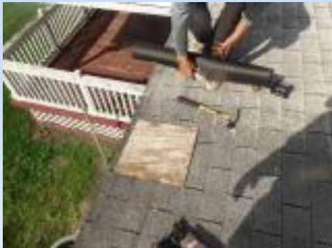
Improper - Board nailed down on top of old roofing
