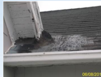
6/8/13 Roof damage photo submitted by HUD
