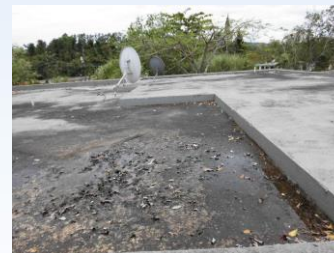
Roof damage inspected by HUD 6-4-13
