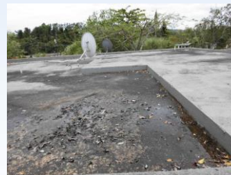
Roof damage inspected by HUD 6-4-13
