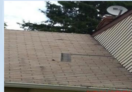
Loose/ missing shingles
