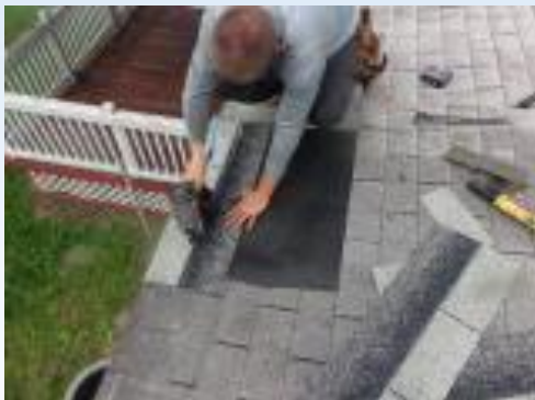
Improper – Shingles being nailed down over old roofing
