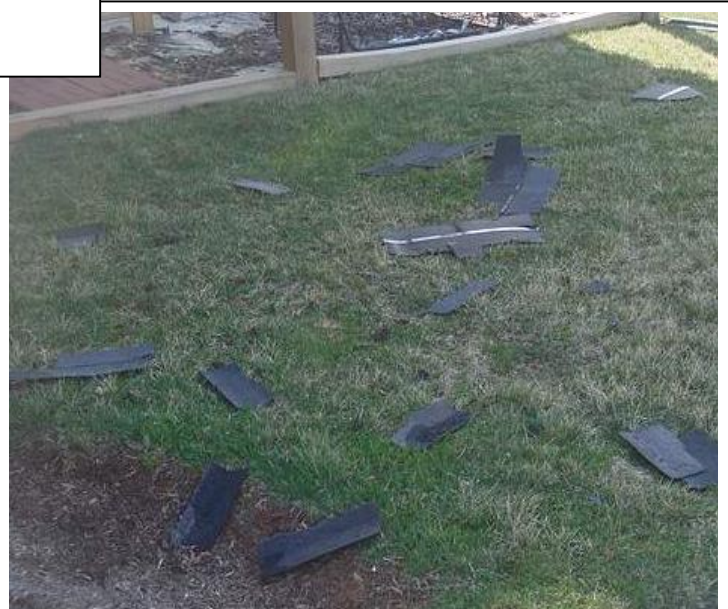
Damaged Shingles on Ground
